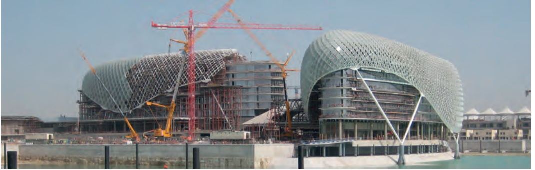
Figure 1. Freeform architecture. The Yas Marina Hotel in Abu Dhabi illustrates the decomposition of a smooth skin into straight elements which are arranged in the manner of a torsion-free support structure. The practical implication of this geometric term is easy manufacturing of nodes (image courtesy Waagner-Biro Stahlbau).
